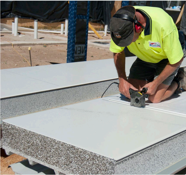
↑ Avoiding thermal bridges in the roofing panels—roofer pictured inserting sawcut gap between internal ceiling and external soffit to obstruct passage for heat conduction.
